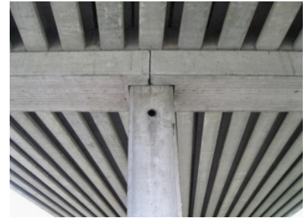
Concrete viaduct at Eger city. Noctules roost in joints between the column and crossbeams [Stephen Morgan]
